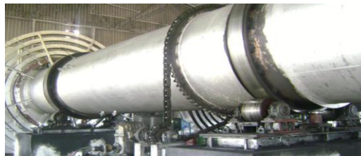
Fig 1. Rotary kiln arrangement
